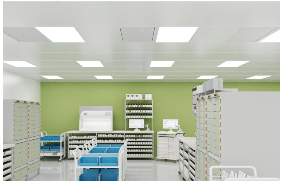
FFU installation in a Pharmacy
